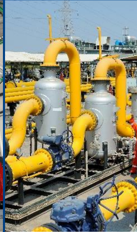
Natural Gas Skid
